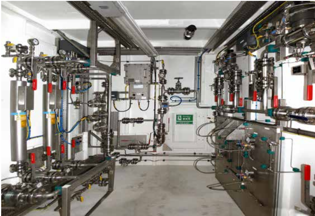
Dual densitometers installed in a sampling and analysis system
